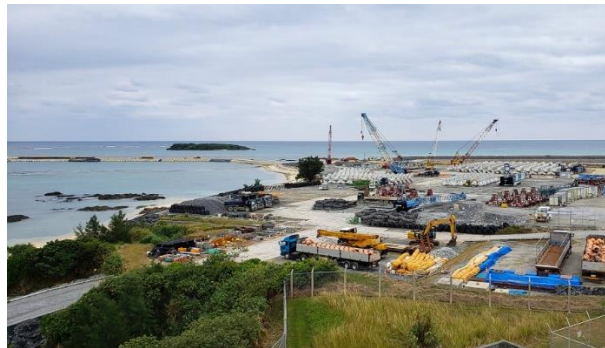
Landfill work for the construction of a Marine Corps runway at Camp Schwab, Okinawa, is seen in January 2020.
